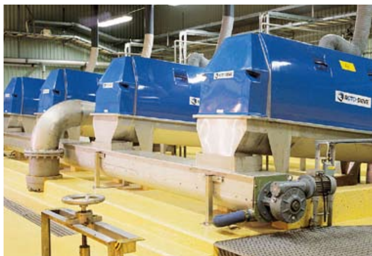
Roto-Sieve drum screens, model 51, installed at Kullavik treatment works in Kungsbacka.
